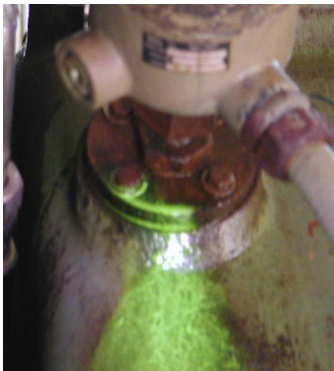
Leak around bolt easily remedied
